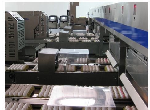
CIJ printers installed on grader
